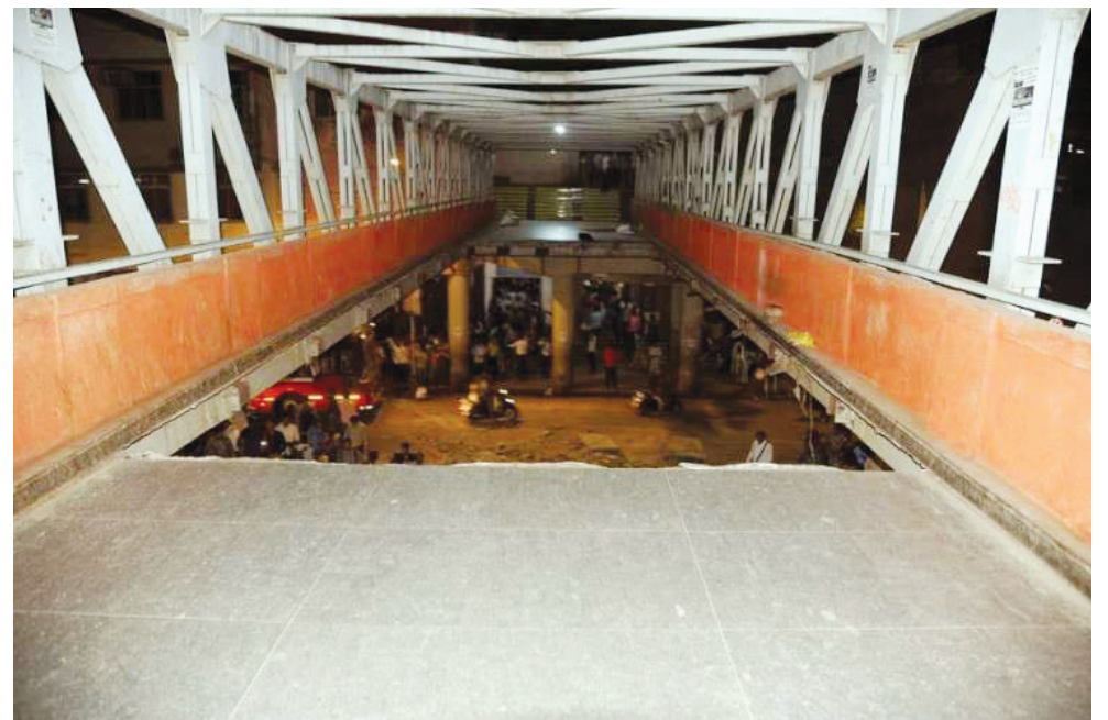
A major portion of the foot overbridge near the CST railway station collapsed on Thursday.
