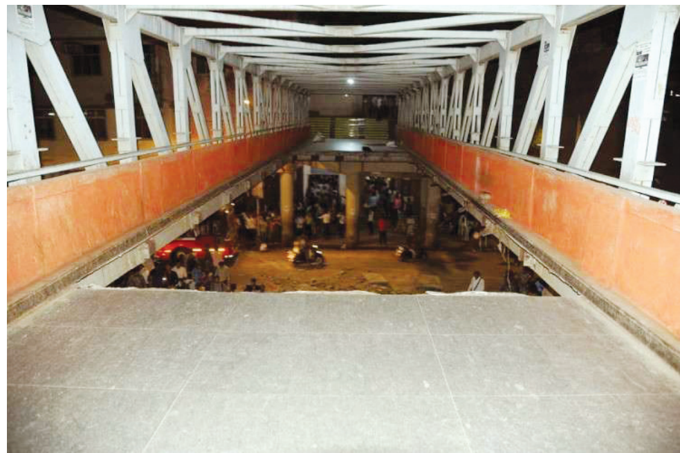
A major portion of the foot overbridge near the CST railway station collapsed on Thursday.
