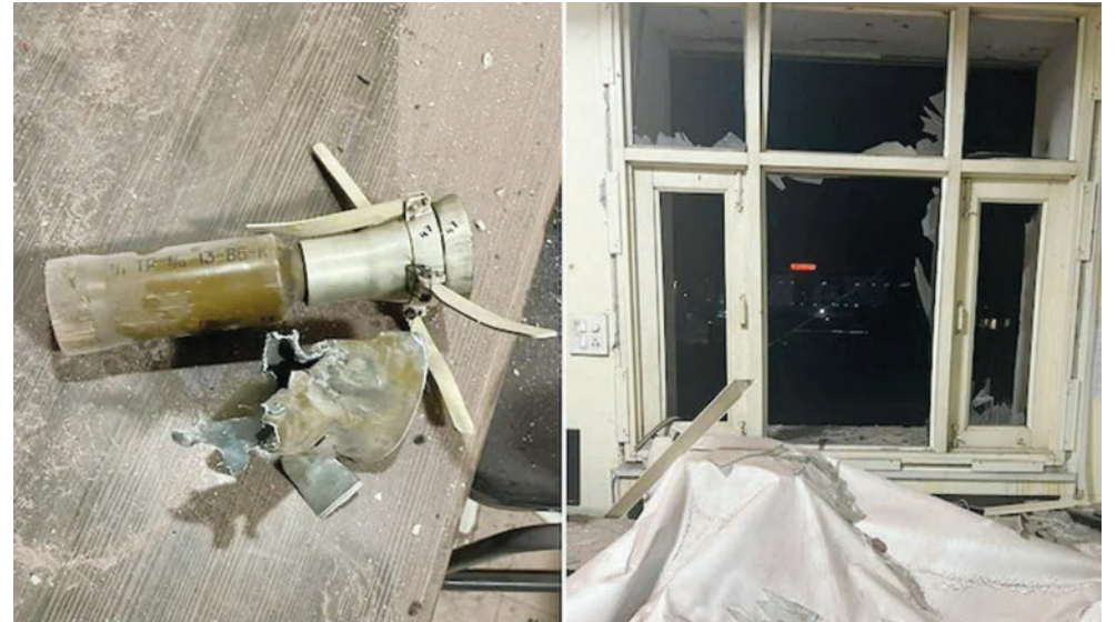
A minor explosion occurred on the third floor of Punjab Police's intelligence office in Mohali on Monday night, May 9, shattering windows and damaging property.
