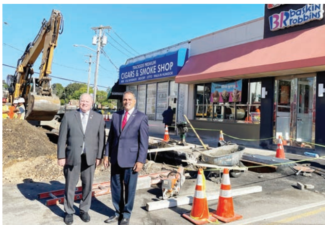
Legislator Drucker and Supervisor Saladino at the site of the Jackson Ave. Streetscape in Syosset on Thursday, Oct. 6.
