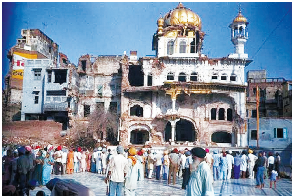
The damaged Akal Takht, the highest temporal seat of Sikhs.
