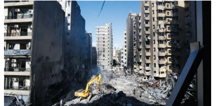
Lebanese first responders use a digger to search under the rubble at the site of an Israeli airstrike that targeted a building. Photo: AFP
